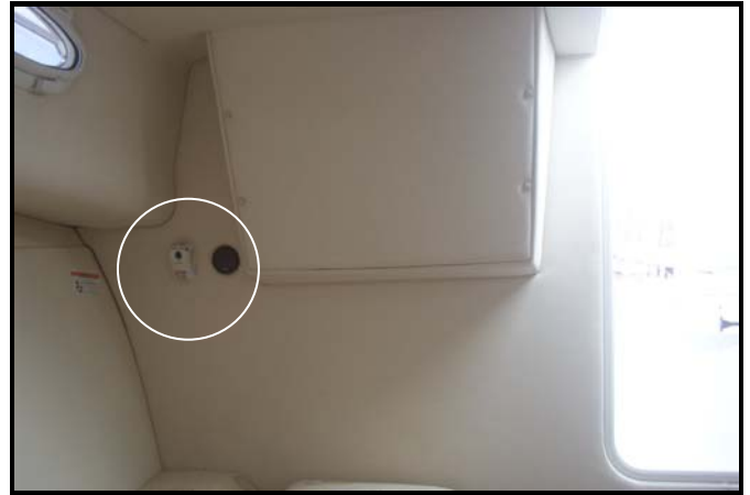
210 Coastal Carbon Monoxide Detector Location
